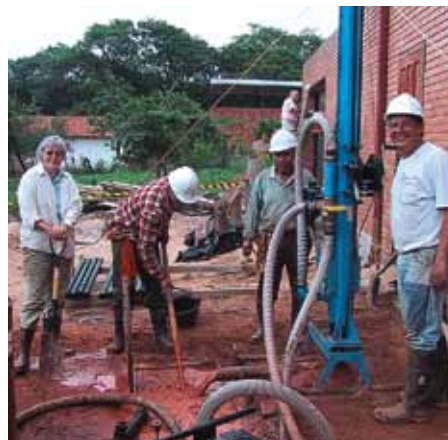
Missionaries Ed and Linda Baker, who serve in Paraguay's interior, drill water wells to assist the existing Methodist churches there and to help plant new churches.
